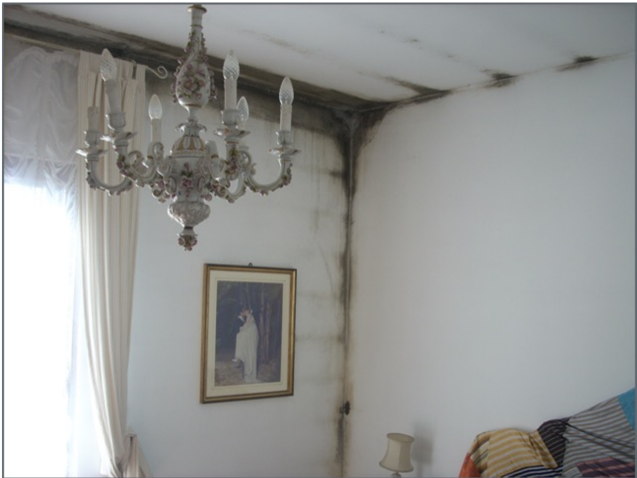
Image 24: Interior of a building afflicted by mold, which resulted from a partial energy retrofit (photo: Damiano Chiarini).
