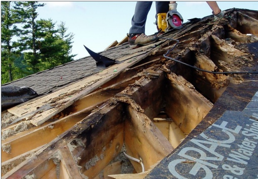
Image 27: Wood rot at the roof. The lack of air tightness allows for warm, humid air to exfiltrate to the outside, carrying moisture from inside the building into the building assembly.
